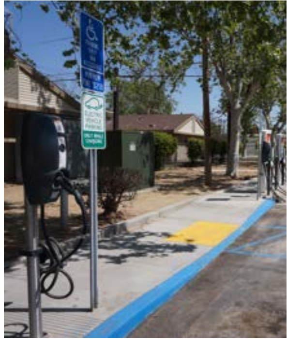
Fig 4.42: CEV Charging Stations at Sierra Terrace
